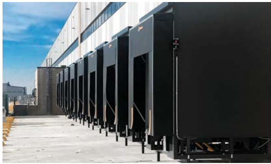
Retractable shelters installed free standing frames and dock houses.
